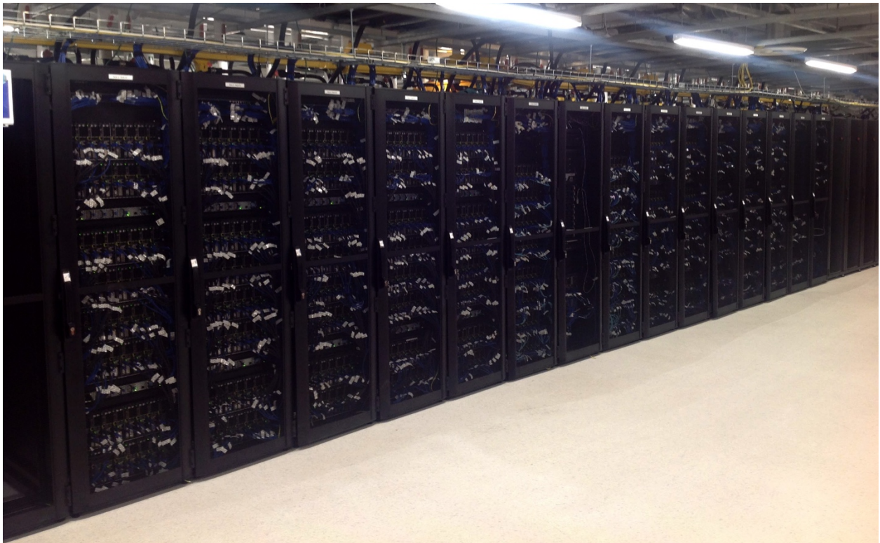
Data centre servers
