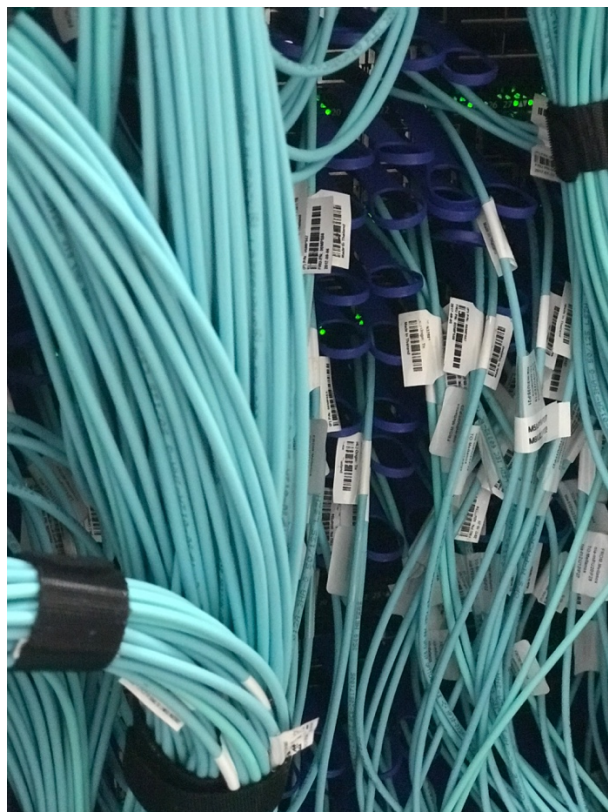
Data centres can require over 40 kilometres of fibre optic network cables.
